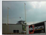
Figure 2.111 UHF antennas used for audio, data or telemetry transmission and reception, like this one at Indianapolis, can be found scattered around large venues.
